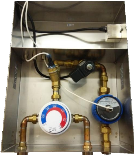
Inside View of BMWMS15
